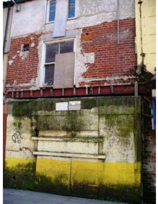
derelict shop on Magdalen Street
